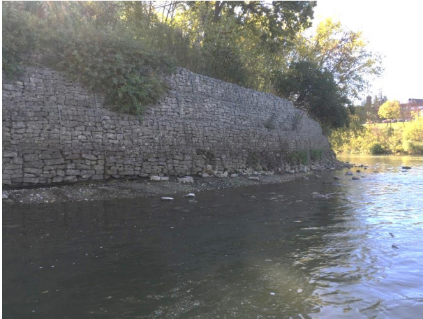
Photo 3-1. Degraded Gabion Baskets at the Forks
