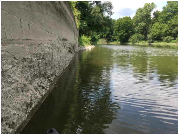
Photo 3-3. Localized Scour at Toe of Rail Embankment Retaining Wall
