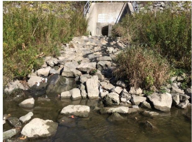
Photo 3-4. Outflow Channel Slope Failure, South Thames
