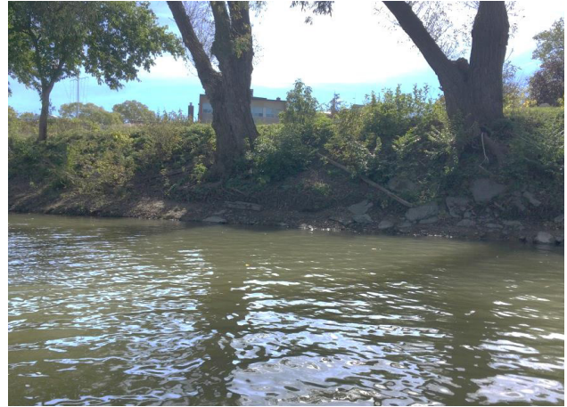
Photo 3-2. Over-steepened Banks, Toe Erosion Downstream of the Forks (left bank)
